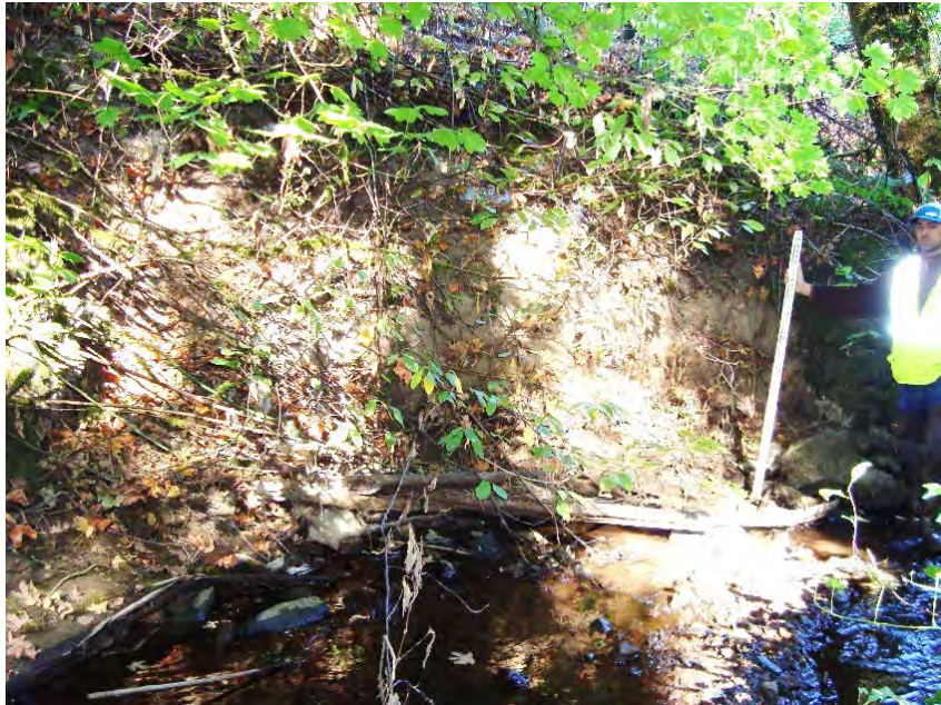
Site location: 175' upstream of SW 105 th Ave. Photo number: H3-5 Description: Left bank failure, missing wall segment adjacent to SW 105 th Ave., outside bend
