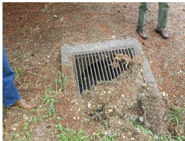
Image 2. Tree debris clogging the ditch inlet at the downstream end of the open channel
