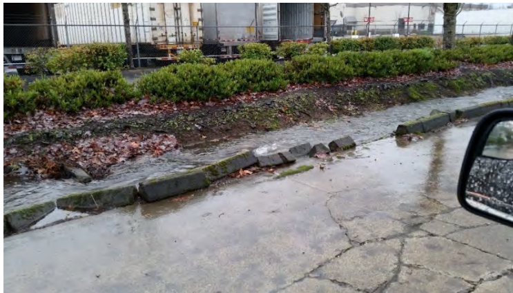
Image 1. Observed flooding of drainage ditch during December 2015 storm
