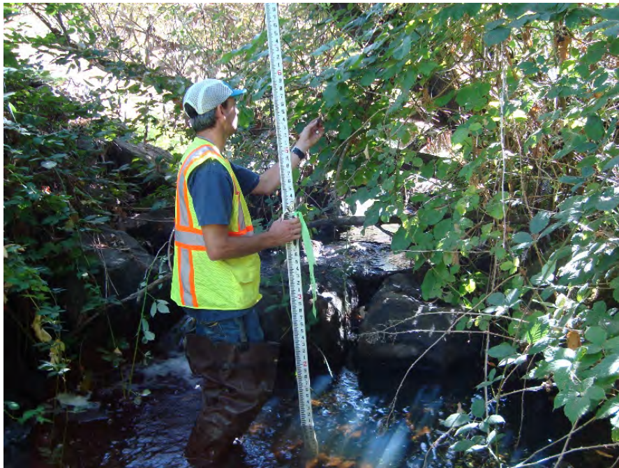
Site location: 100' downstream from SW Industrial Way Photo number: H2-13 Description: Rock drop pool formed by rip-rap energy dissipation at culvert outfall
