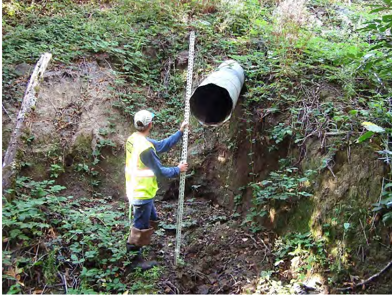
Photo 1. Hanging culvert on north side of Saum Creek Reach #3 in location of hillslope failure (September 2017)
