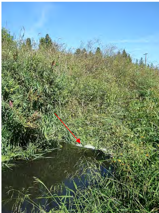
Site location: 400' upstream of SW Nyberg Lane Photo number: N1-6 Description: Looking downstream at top of beaver dam. Red arrow points to top of dam. Drop is approximately 3 feet.
