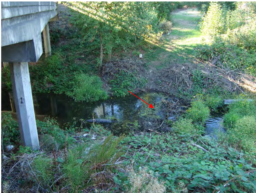
Site location: Nyberg Creek on downstream side of SW 65 th Ave (east side) Photo number: N1-12 Description: Photo taken from south side on 9/11. Red arrow shows debris removed from beaver activity.
