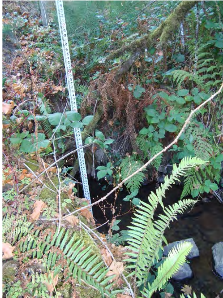
Site location: Culvert under SW 105 th Ave (downstream side) Photo number: H3-1 Description: Looking upstream at SW 105 th Ave. culvert crossing from west side of SW 105 th Ave.
