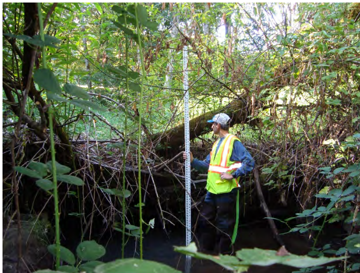
Site location: Between SW 55 th and SW 56 th , near I-205 Photo number: S2-4 Description: Channel spanning debris blockage, ~4' above channel bed, looking south and upstream
