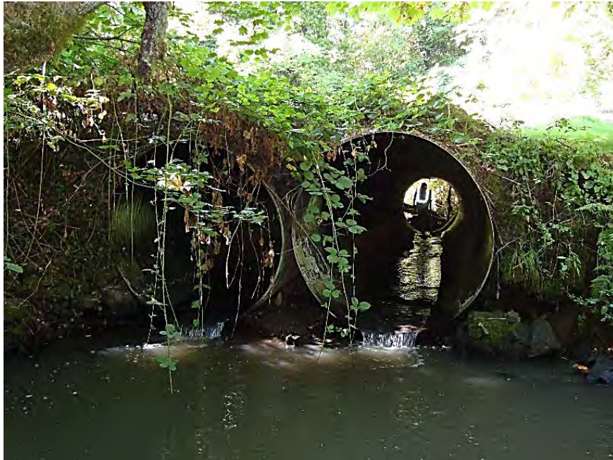
Site location: SW Halcyon Rd. culvert crossing Photo number: S1-9 Description: Looking upstream- twin 6' culverts, plunge pool on downstream end
