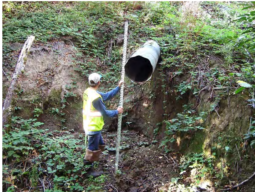
Image 1. Perched outfall from Blake Street with severe bank failure
