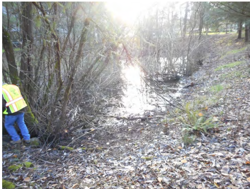
Image 1. Vegetation and cottonwood trees growing in the water quality facility
