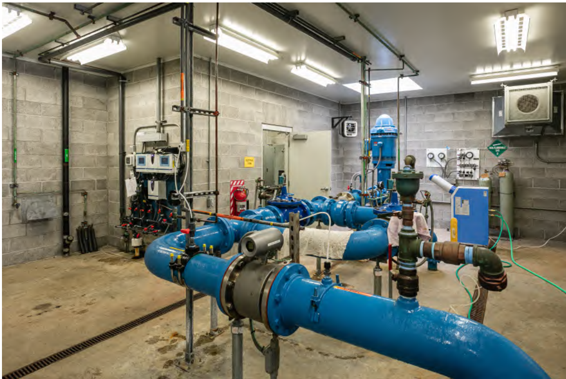
Aquifer Storage and Recovery (ASR) site
