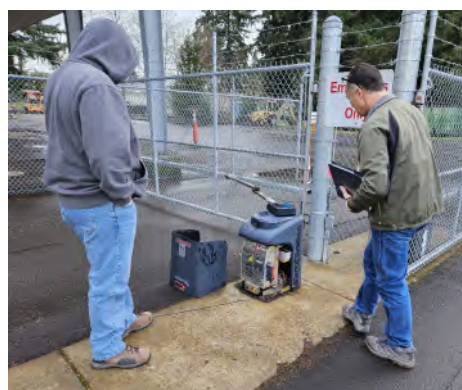
Electrical Component Failure
