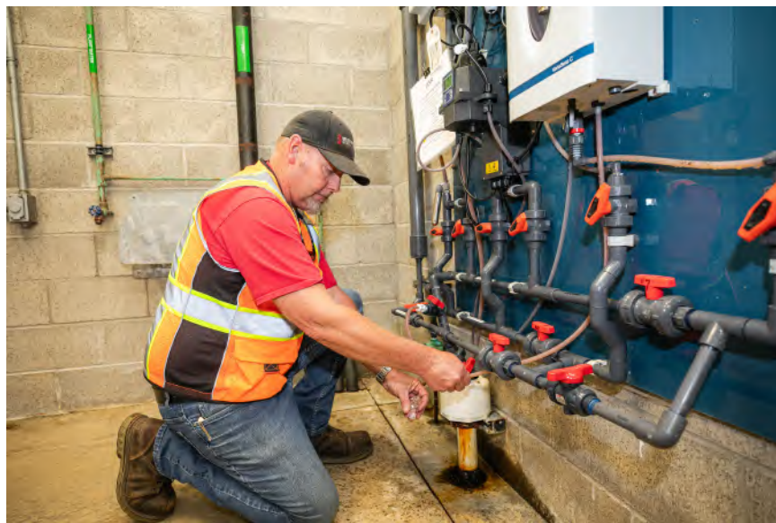
Testing the chlorine levels in the water system
