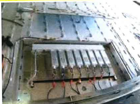
Service access centered at bottom for electric hook-up and maintenance at bottom/back of sign.
