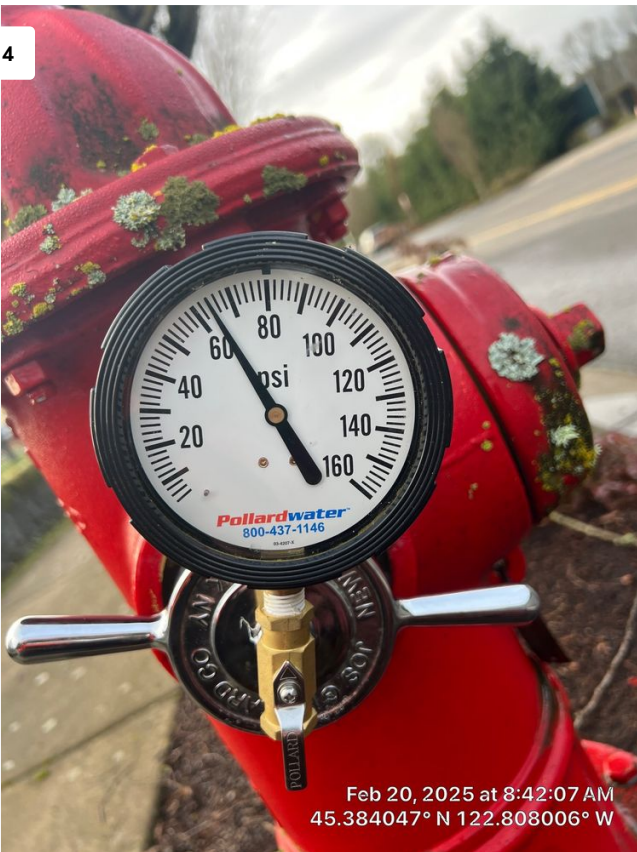
The static psi of the gauge/residual hydrant at 64 psi.
