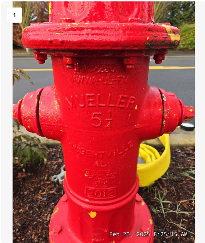
The flow hydrant, a Mueller 5 1/4.
