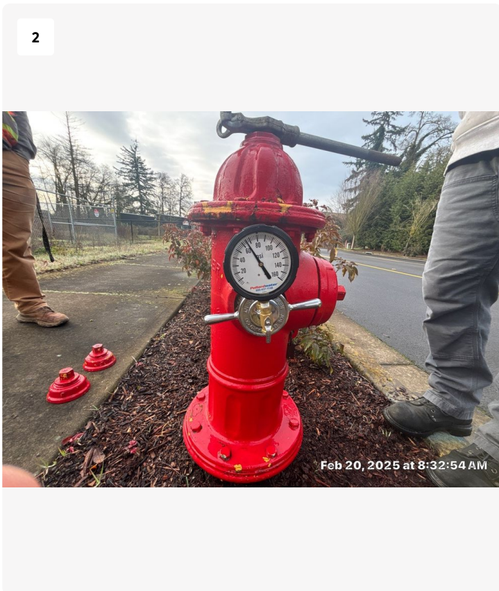
The static psi of the flow hydrant at 66 psi.
