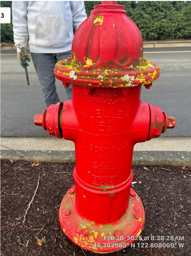
The gauge/residual hydrant, a Mueller 5 1/4.
